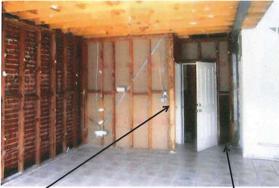
Damage to studs close to entry/sub nest location point on ground floor
