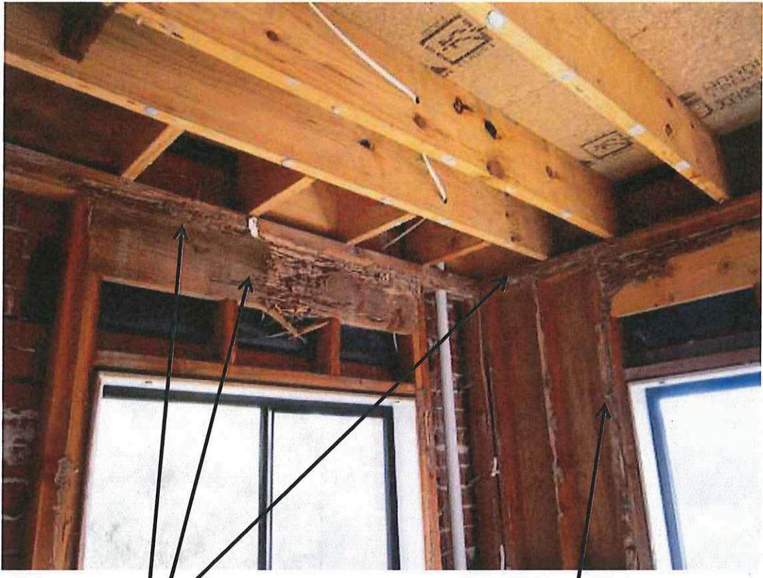
Damage to beam/window lintel on ground floor level Damage to studs on ground floor level
