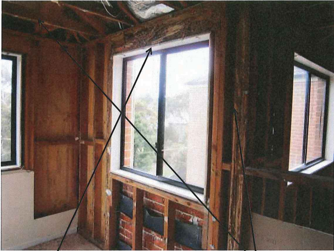
Damage to lintel above upstairs bedroom window, as originally located in December 2010
