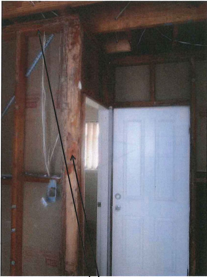
Closer view of damage to studs close to entry/sub nest location point on ground floor. Shows travel up the stud and along the top beam.
