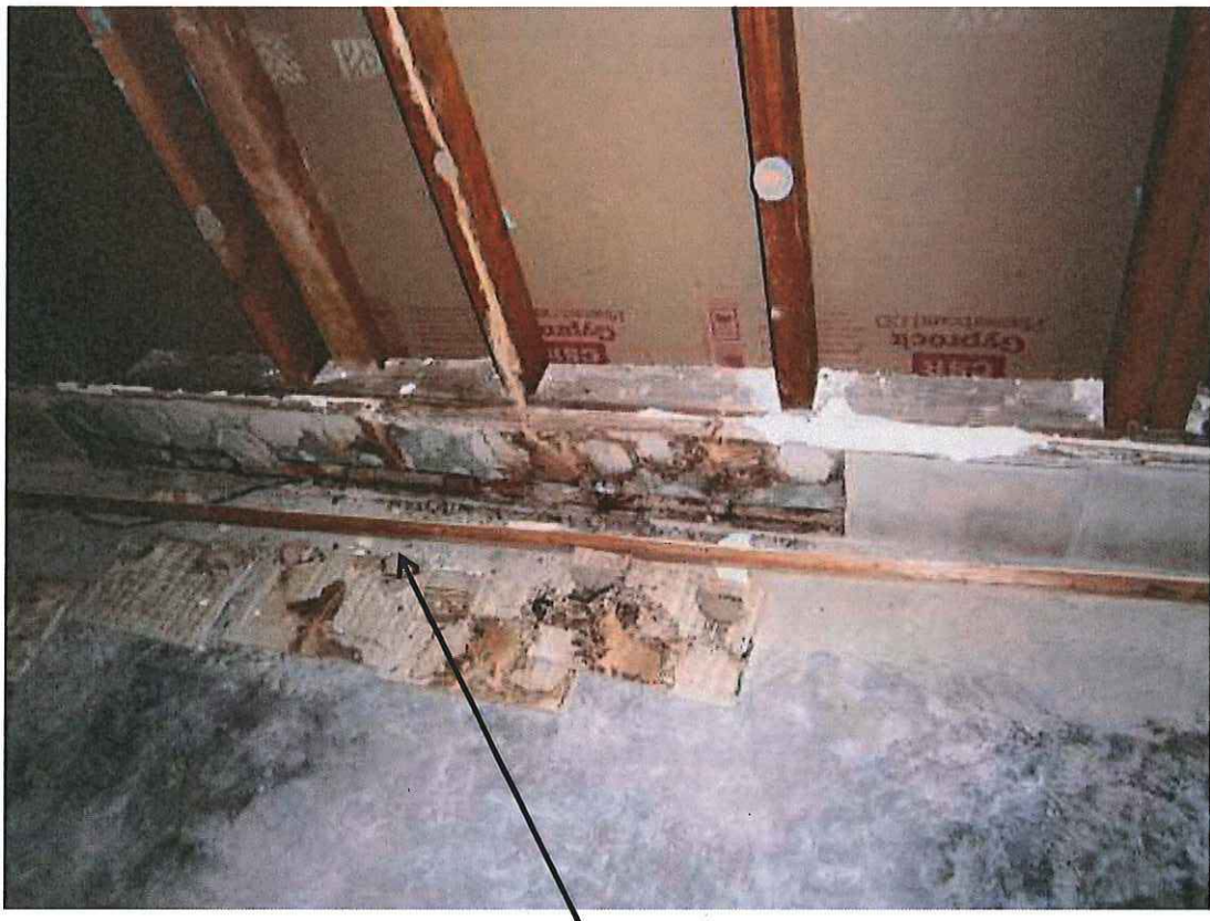
Closer view of location of entry point at slab joint in garage
