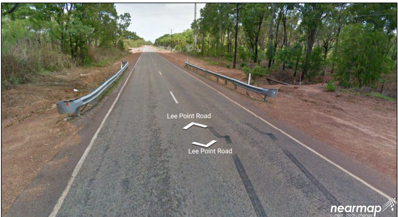
Figure 11. Culvert cross of Lee Point Road 115m south of the Lee Point Resort (Nearmap 2016).
